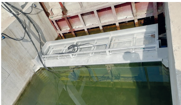
Figure 10 Drainage of the overflow structure and preparing of the assembly (top); finished system consisting of hydraulically driven raked bar screen and flushing gate below waterline (bottom) 图 10 溢流结构的排水和组装准备工作 (上)；由液压驱动的格栅系统和位于水位线以下的冲泄闸门组成的成品系统 (下)
