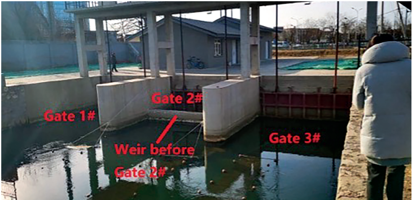
Figure 8 Overflow structure Yudai River Channel with gates (old state); overflow weir in the center 图 8 带闸门的玉带河溢流结构（水泰和设备安装前）；溢流堰位于中心
